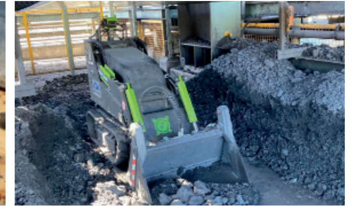
Power plant maintenance / Mining Industry
